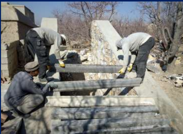
Builders are shown constructing one of the nearly 70 apple cool rooms constructed by CHAMP during 2013. Cool rooms offer farmers the ability to hold back portions of their harvest to sell when market conditions improve in the months after harvest.
