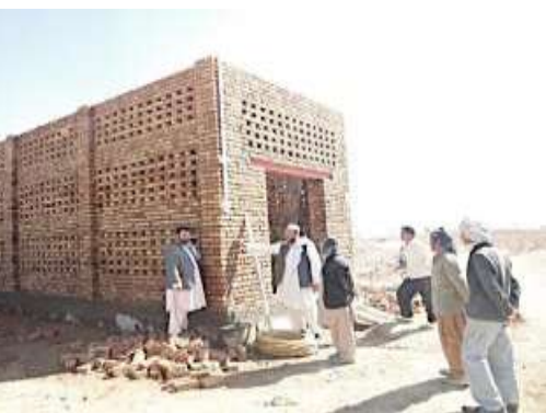
A raisin drying facility is shown in the early phases of construction in Ghazni Province. CHAMP constructed 121 of these facilities in 2013.
