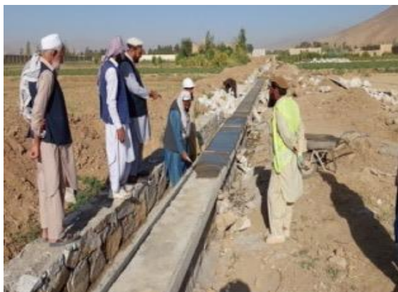
Workers install stone masonry on one of AMP's five canal and karez rehabilitation projects.
